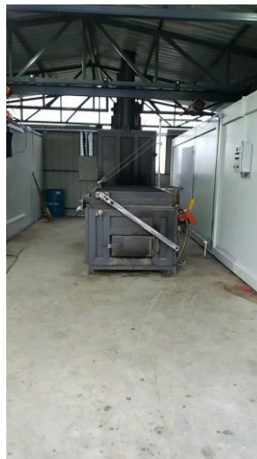
Fig. 1. Incinerator INCINER8 Model I8-250, on the right side there is a sanitary and office container, and on the left side there is a refrigerator of the container type.
