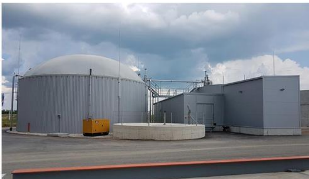
Fig. 4. Biogas power plant (300 kW) in the Hrastin village
